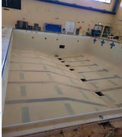
PE Building, Pool Investigation Project: Ongoing, Arch/Engr Contract to be executed by Spring '24
