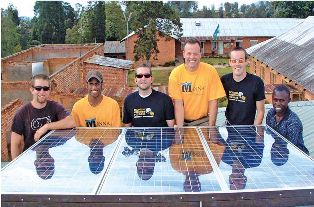
© BERNARD AMADEI Engineers Without Borders volunteers help erect a solar energy project for a hospital in Rwanda.
